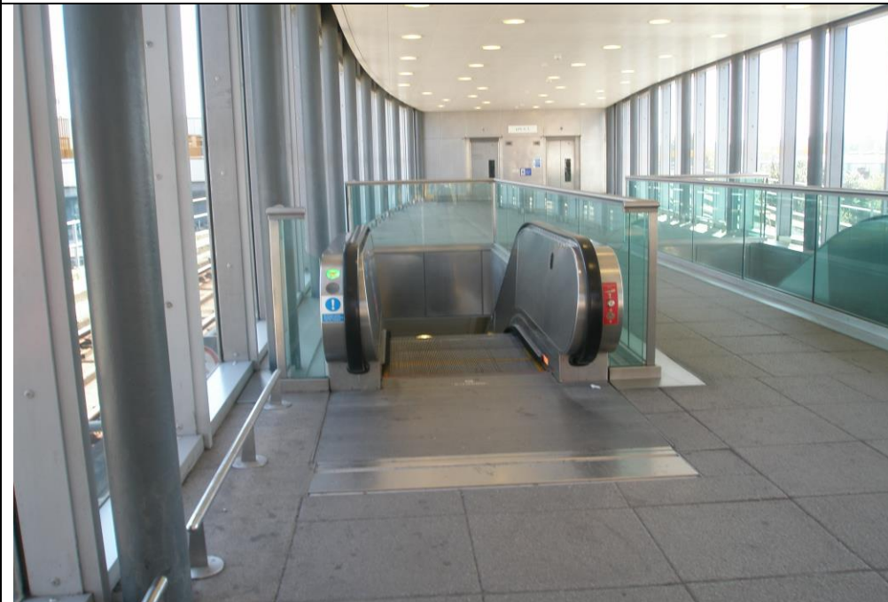
Escalator 1 Platform Level
