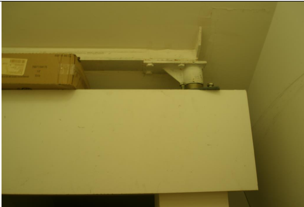
Escalator 1 Intermediate Support -Store 1/411
