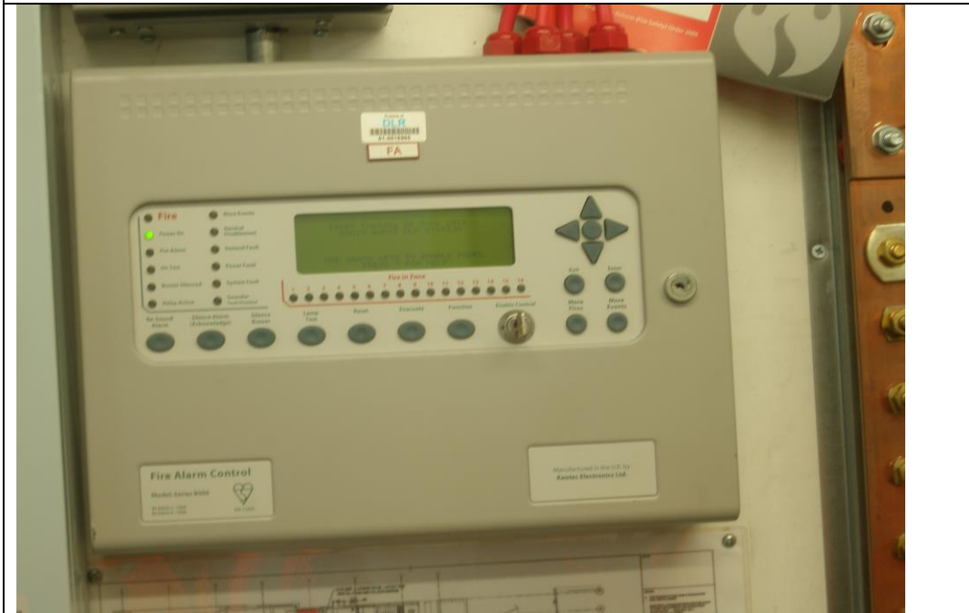
KENTEC Fire Panel, L.V. Switchroom 1/662
